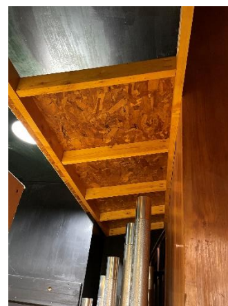
This is a photo of the overhead cover that was built to protect the pipes from water damage.
